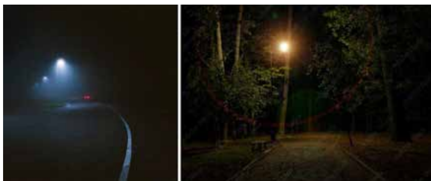
Figure A.2.9 – Street lighting lanterns
