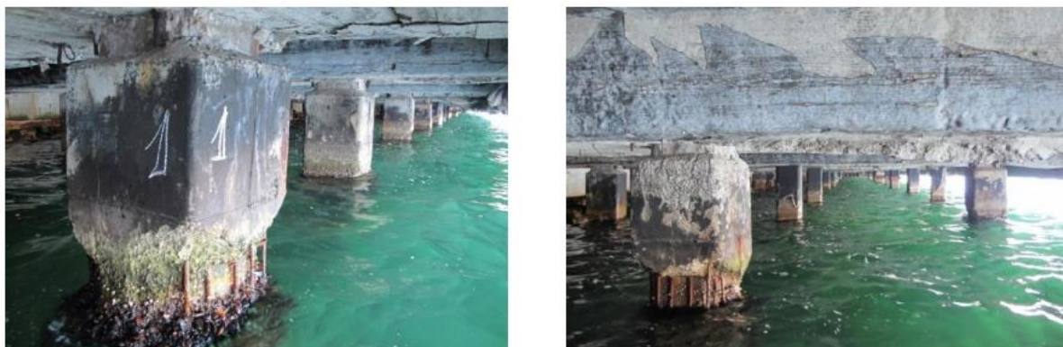
Fig. 1. Defects and damage to reinforced concrete structures
