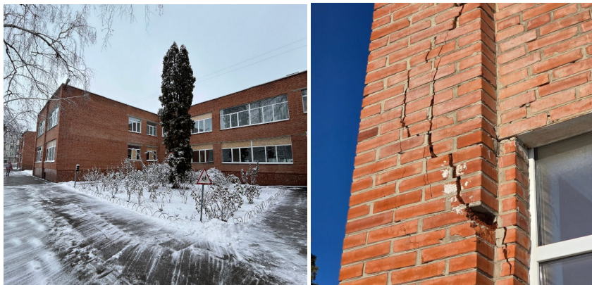
Figure 3.13 – Damage to preschool educational institution No. 81[88]
