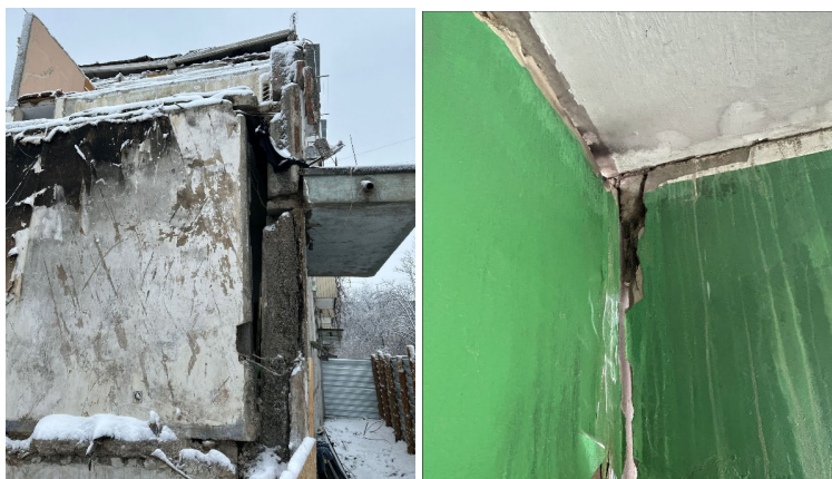
Figure 3.14 – Opening of seams and damage to the joints of the panels of the entrance group of the first entrance
