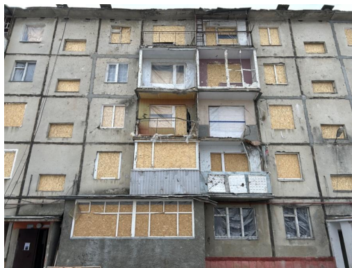
Figure 3.12 – Damaged by debris and blast wave, the facade of a house No.5 [89]
