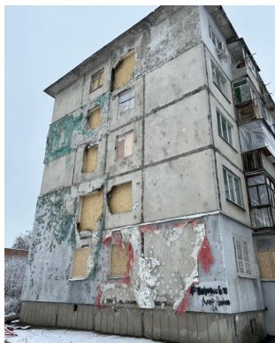
Figure 3.11 – Damaged façade of a house No.7A [89]
