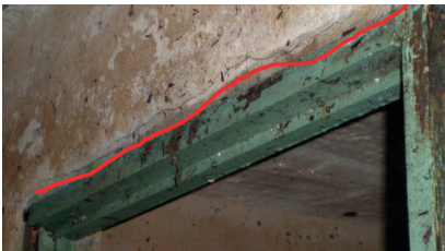
Figure 3.3. Formation of cracks in load-bearing structures above door openings
