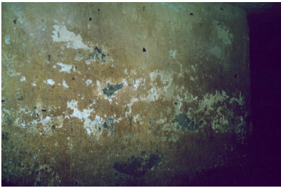
Figure 3.1. Destruction of the protective concrete layer of walls and slabs
