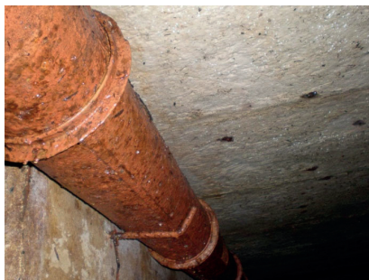
Figure 3.6. Moisture condensation on the surfaces of reinforced concrete structures
